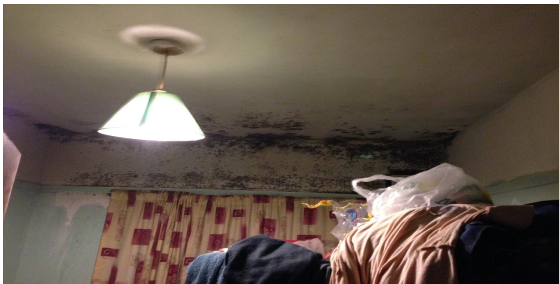
Picture 2: Mould in the rooms at the property as a result of overcrowding
