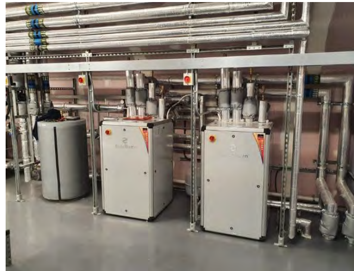
Commercial scale Ground Source Heat Pump systems have also been used for years in many types of non-domestic buildings
