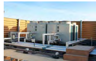
Communal rooftop air source heat pumps (Source: Mitsubishi electric)
