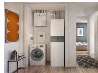
Individual heat pump in each dwelling (Source: Dimplex)
