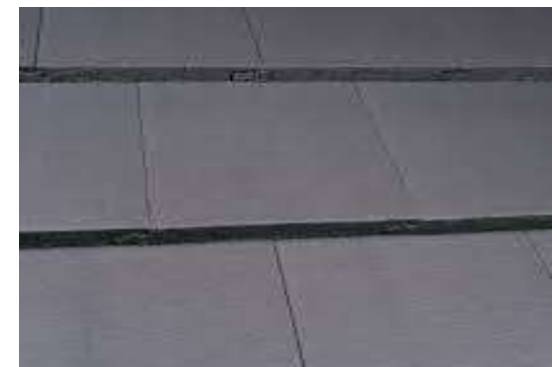
Concrete roof tiles - not supported
