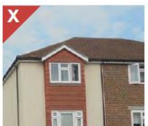
Figure 2.19e: Pitch of roof appears too shallow in relation to mass of building.
