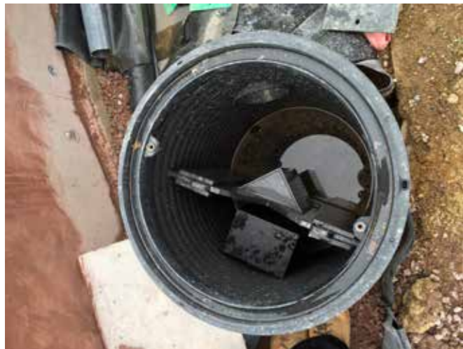
Orifice flow control chambers such as this one by Controflow are simple, reliable, cost-effective and easy to maintain.
