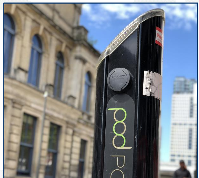
Freestanding electric charging point, Stratford High Street
