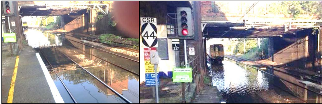
Figure 2 Photographs of flooding at Manor Park Station (19/09/2014)
